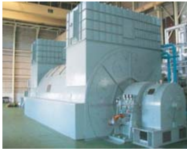
Short Circuit Generators (Closer View)
