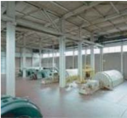
Short Circuit Generators at High Power Test Laboratory
